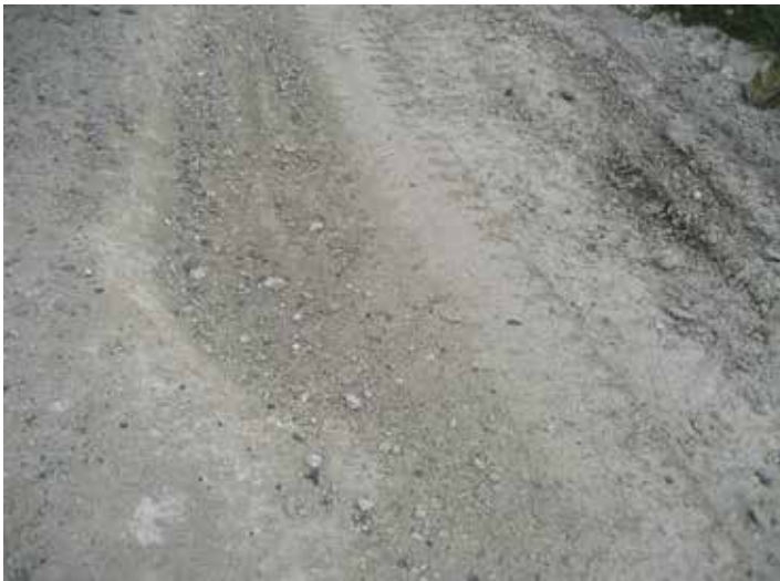
Pavement showing a soft spot
