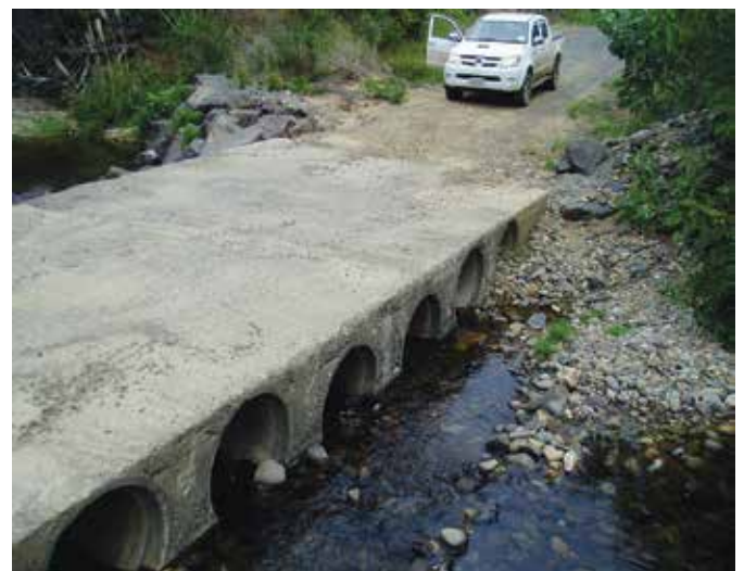
This battery culvert provides for fish passage
