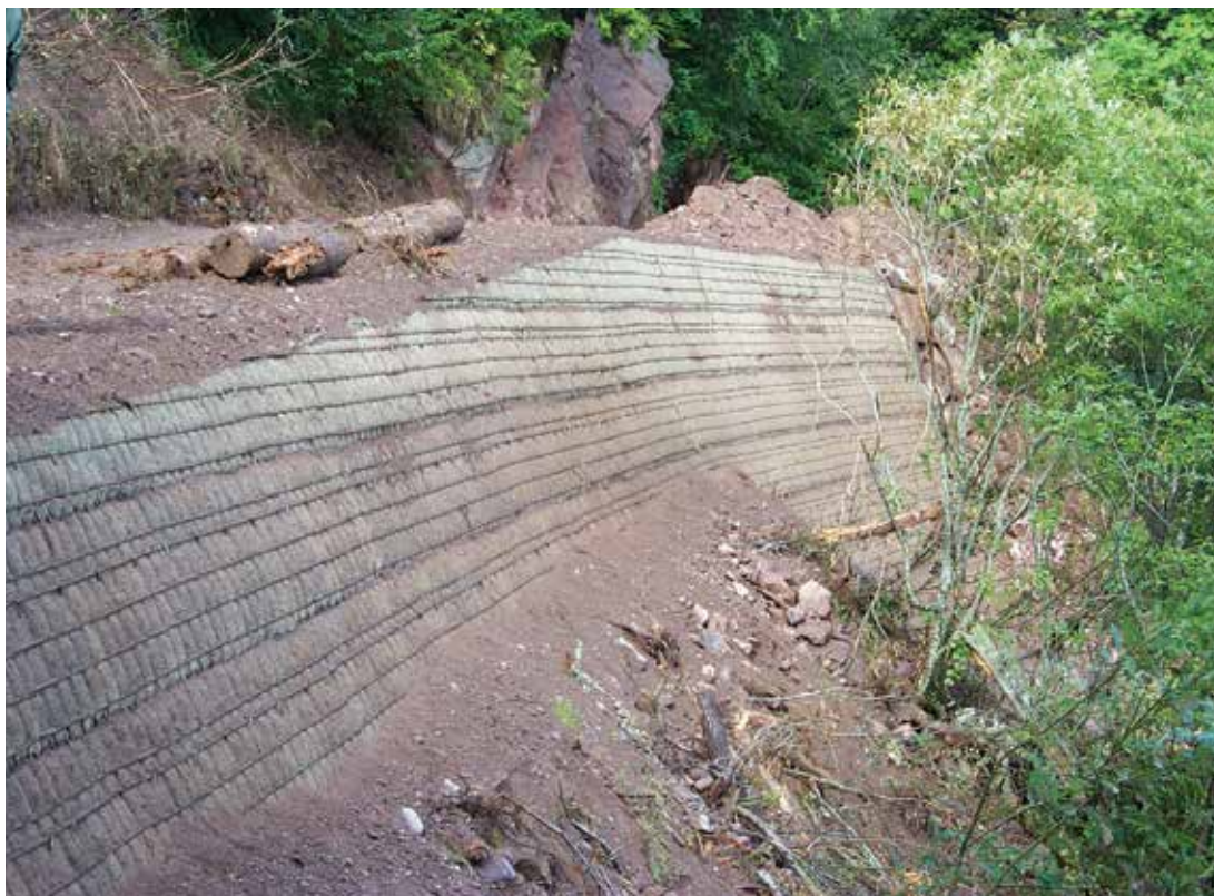
MSES fill slope of a forest road
