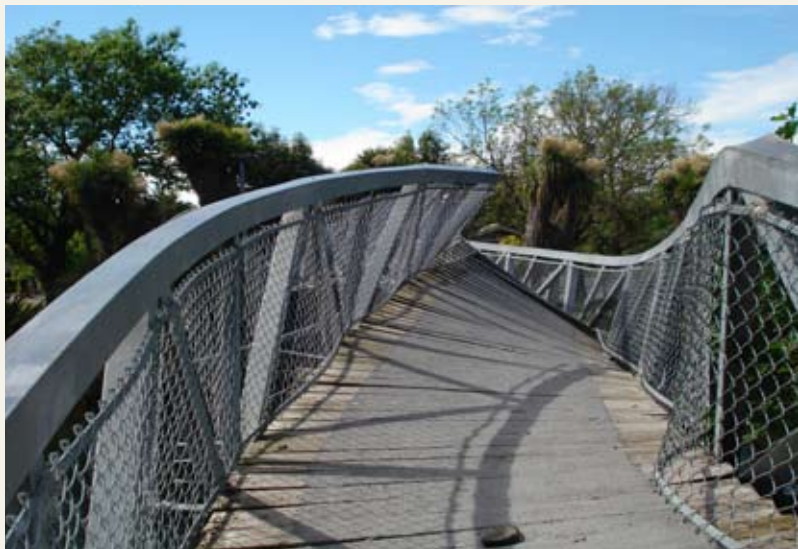
The forest and wood processing industries have offered to rebuild at their own expense the footbridge over the Avon River at Avonside in Christchurch (shown above). Already, offers of support have come from forest owners, processors, fabricators and contractors, architects and engineers. "We want to make a useful contribution to the rebuilding of Christchurch after all its citizens have endured," says Jason Guiver, director of the NZ Wood Design Advisory Centre. "Ideally it will have some heritage qualities in keeping with the general tone of the city ... something that local people can identify with." A concept design is being developed as a basis for consultation with the local council and community. The rebuild is expected to be completed in 2011. Wanting to contribute or participate? Contact jason@nzwood.co.nz
