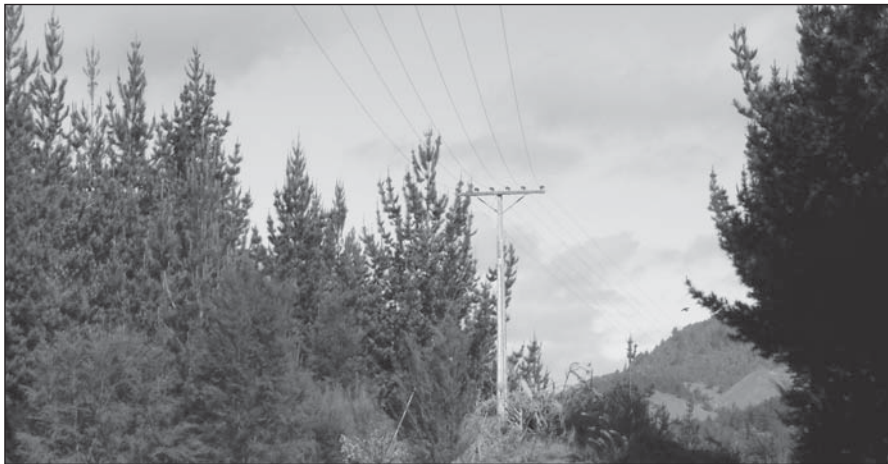
Easement agreements are essential when lines are upgraded The more power going down the line, the greater the potential liability for an outage
