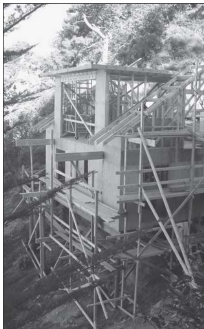
The greatest concern for the public must be that the new standards will not ensure their new homes will be moisture-proof
